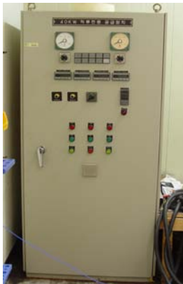
Fig. 3 DC power source
