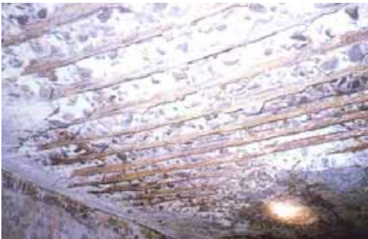
Photo 1 Example of biochemical corrosion in sewer
