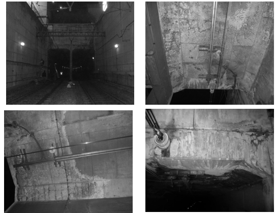
Fig. 9 The Views of Exit of tunnel B and Scaling By Freezing and Thawing
