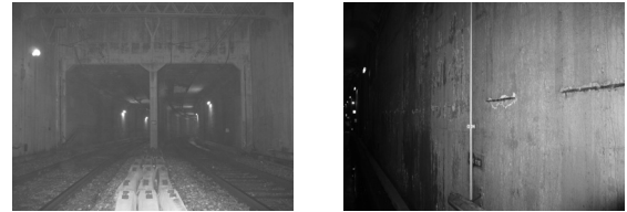
Fig. 4 Tunnel A Exit(Left), Condensation and Exposed Rebar(Right)
