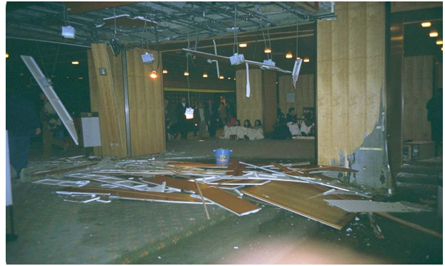
(Fig. 1) Nonstructural Earthquake Damage in Oriental Hotel Lobby in 1995 (Photo: Western Washington University) [1]
