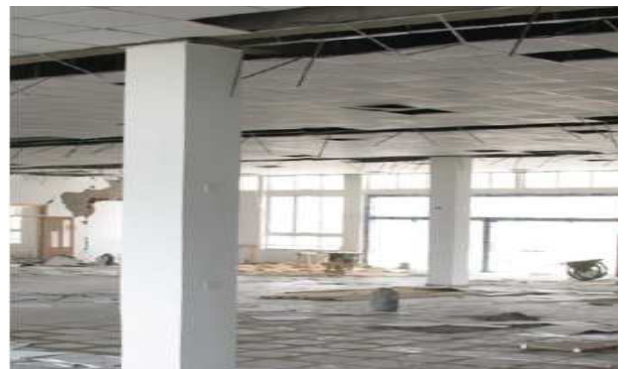
(Fig. 2) Nonstructural Earthquake Damage by Sichuan Earthquake in 2008, Photo: Report on the 2008 Great Sichuan Earthquake, 2009) [3]
