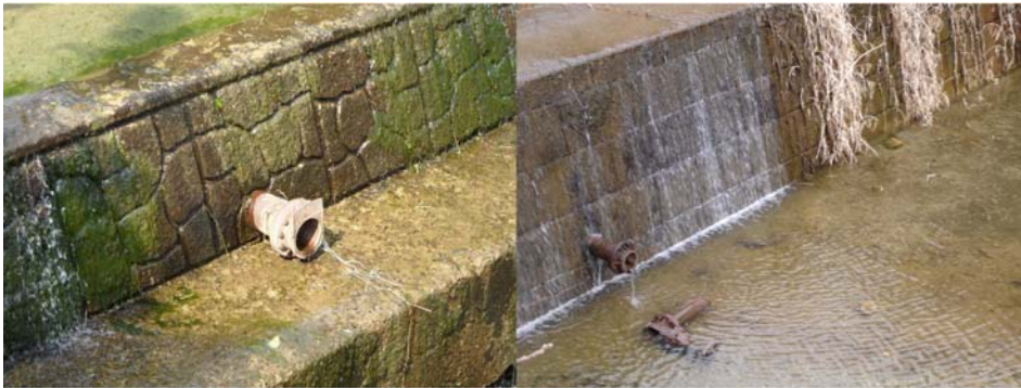
Fig. 7. Corrosion of the weep hole.
