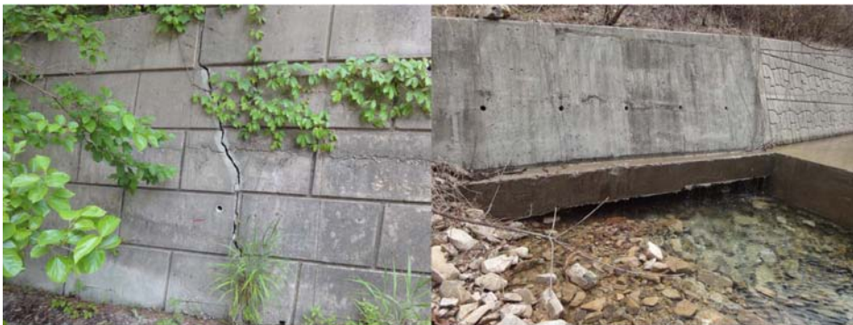
Fig. 8. Crack (left) and scouring (right) under the side wall.
