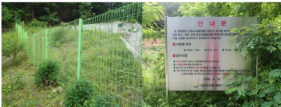
Fig. 11. Safety fence (left) and sign board (right) of the check dam.
