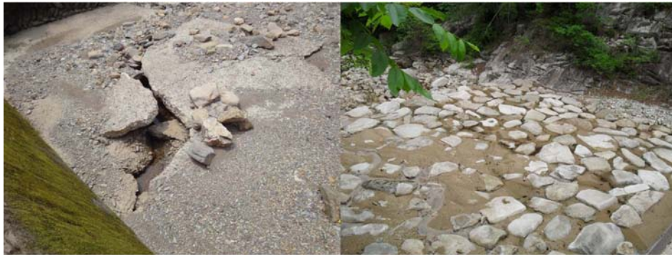
Fig. 5. Destruction of the apron (left) and its restoration (right).
