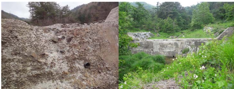
Fig. 4. Concrete deterioration of the main dam body.
