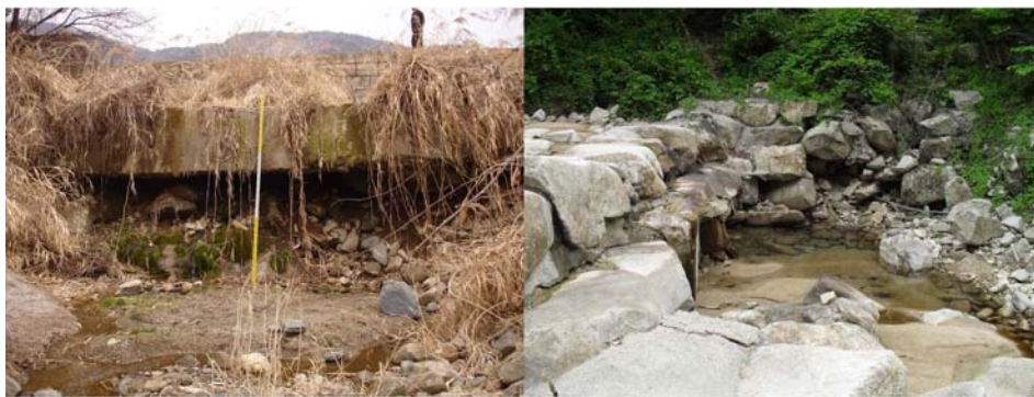
Fig. 6. Scouring in the apron down-side-end.
