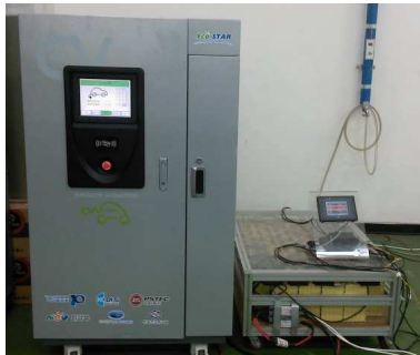
(a) Charging test setup for 320V 20kWh LiFePO4
