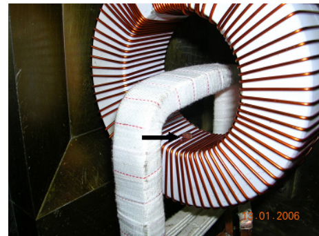
Fig. 3. VL on the low-voltage side of CRCT
