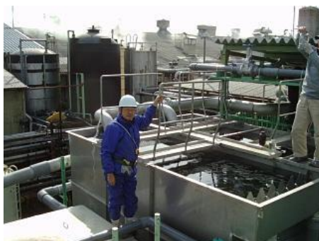
Fig. 5. The effluent processing system.
