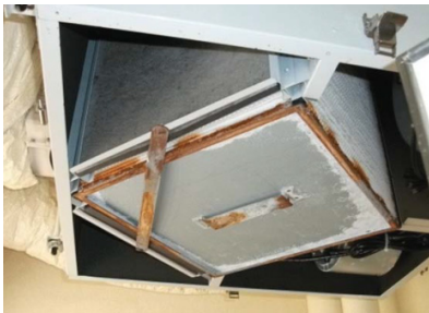
Fig. 1. Corrosion of a heat-recovery ventilator by dew condensation.
