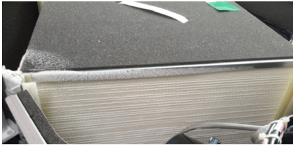
Fig. 10. A photo of freezing in case of -20^{\circ}\text{C} of OA temperature and 0^{\circ} open of recirculation damper.
