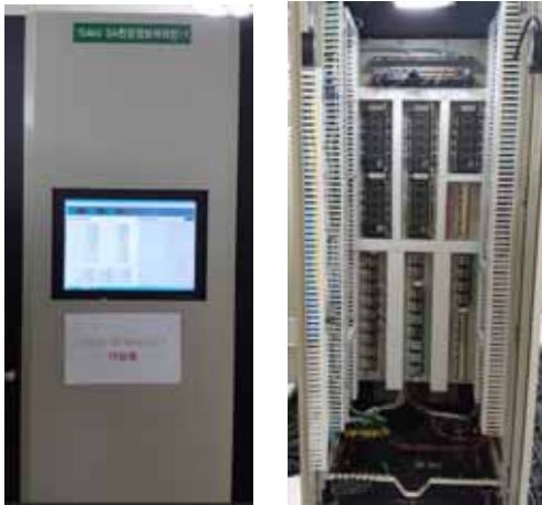
5. IEC 61850 Fig. 5. Installed IEC 61850 based field information processing panel
