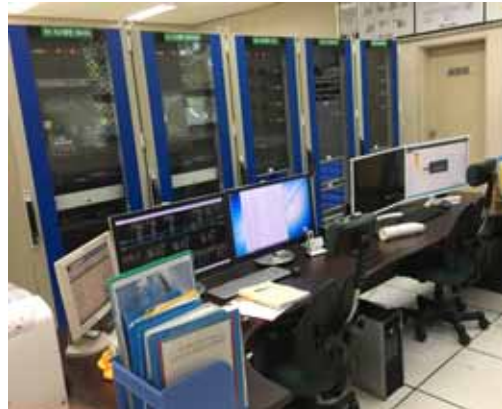
6. IEC 61850 SA HMI Fig. 6. Installed IEC 61850 based SA operating system and HMI
